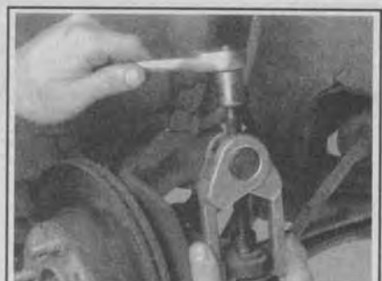
Fig. 58 A tie rod puller is the correct way to remove the tie rod without damaging parts
